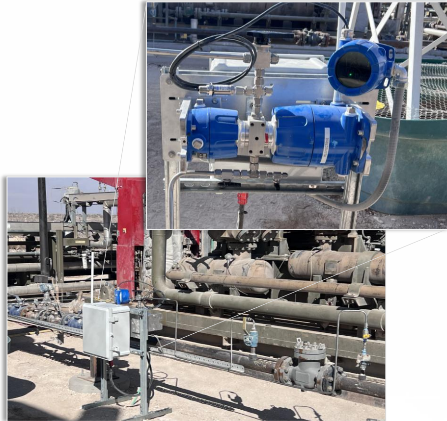
XSPCT Analyzer Installed on customer location in the Permian Basin
