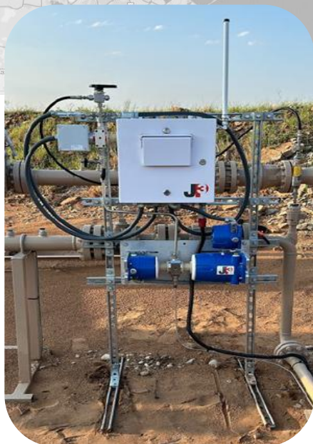
No Shelter, No Calibration Gas, Remotely/Continuously Monitored
